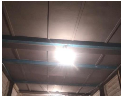
CEILING BATON FOR LIGHTS
